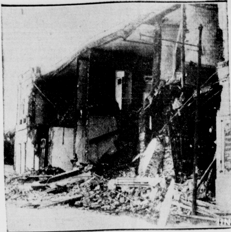
Peace may reign in the Western Hemisphere, but Chile nevertheless had its share of death and destruction this week. Above is shown damage done by an earthquake at Talca, one of the many Chilean cities which were partly demolished. Many thousands of lives were lost.
