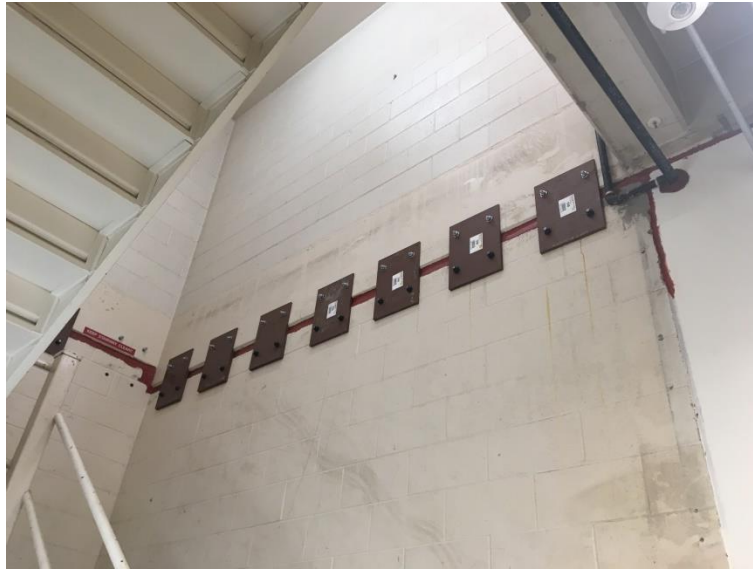
Figure 2.21. Detachment of masonry wall from the structure.
