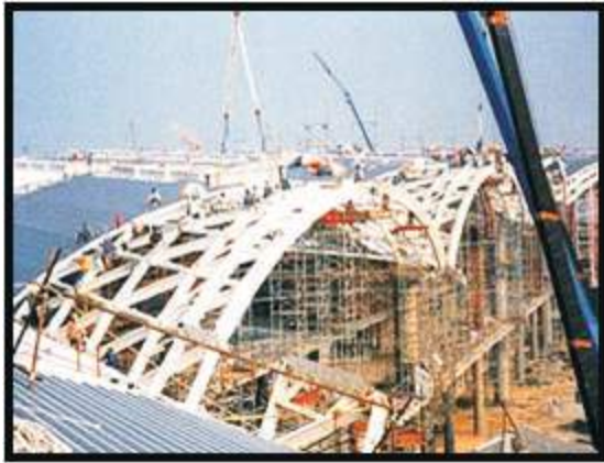
Gambar 10. Proses pemasangan rangka baja (atap) di Chek lap kok Airport diperlukan mobil derek
