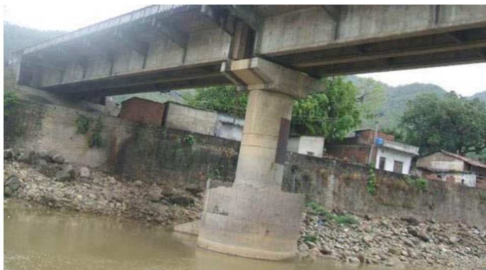
Figure 1.2. Scour around bridge piers on the Tinau River, Nepal (Shrestha, 2015)
