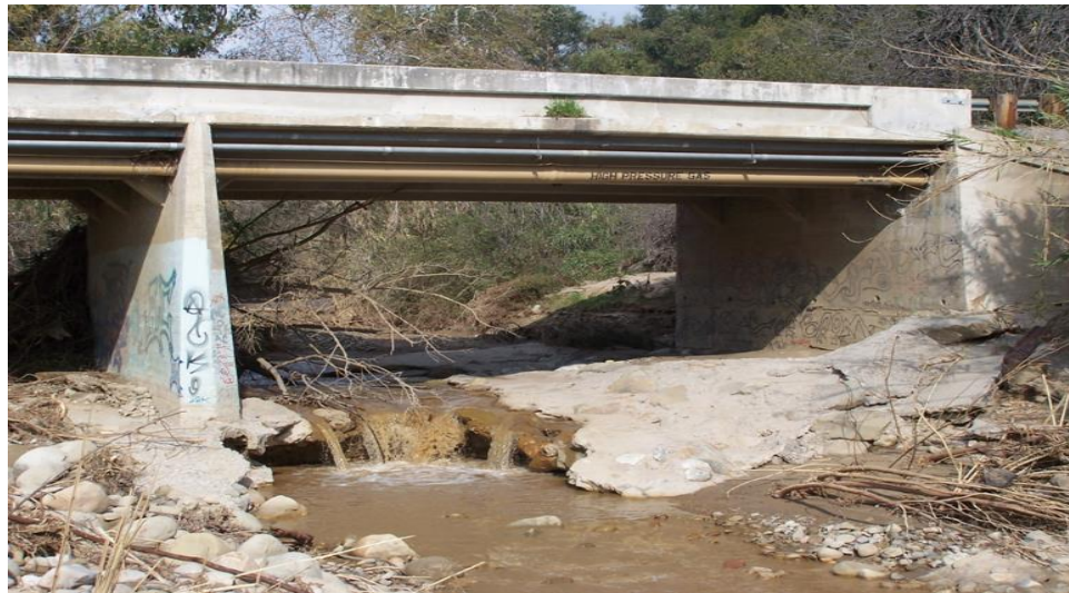
Figure 1.1. Ellsworth Barranca Bridge experiencing problem due to scour in Ventura County, California (California Department of Transportation)
